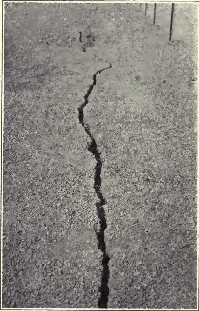
AN EARTH CRACK
